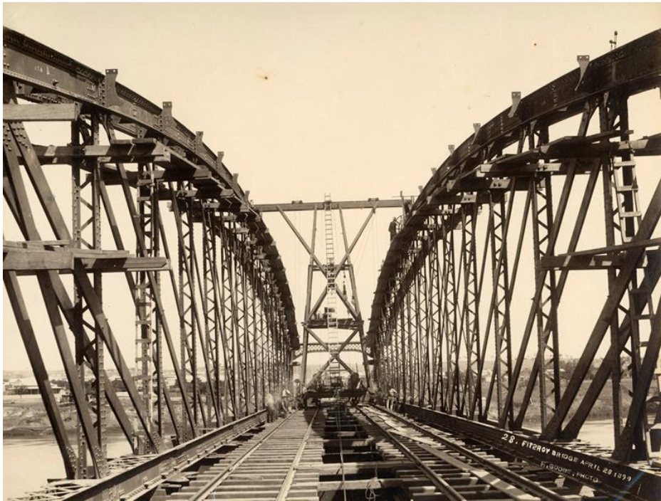
Construction of the Alexandra Bridge, Rockhampton, Henry Goode. Courtesy Queensland Museum Network Collection
